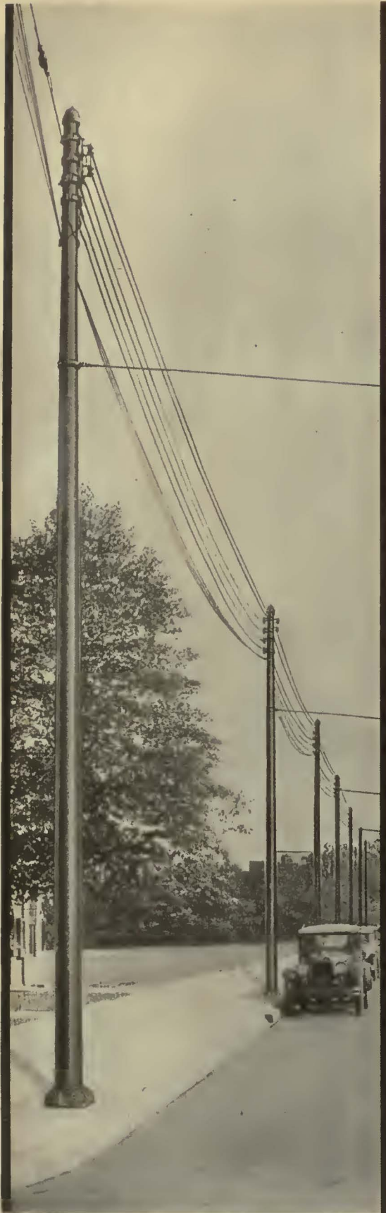
Monotube Pole with ornamental base used for distribution lines and trolley span wire support.
