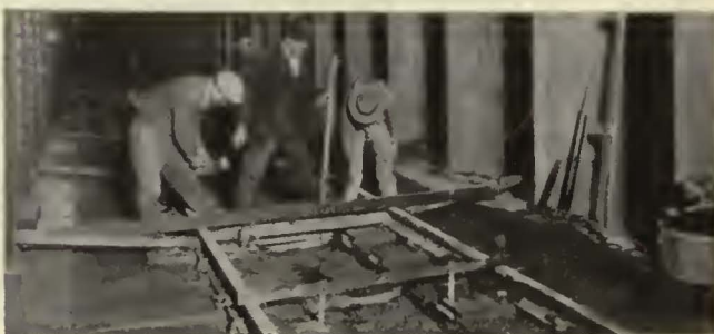
Checking line, grade and gage of track before the first set in the concrete
