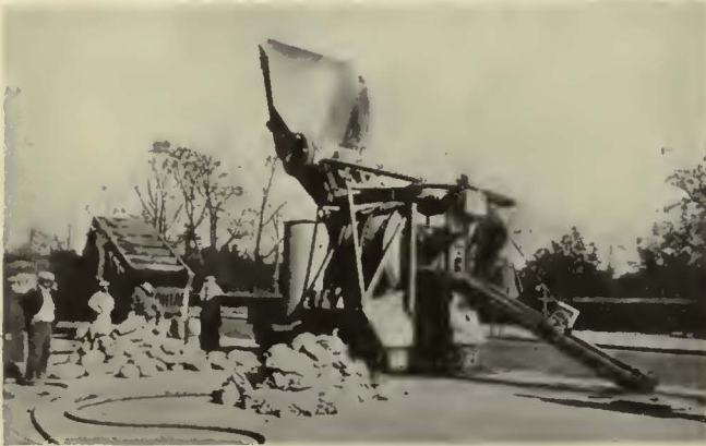
Concrete mixer obtains batches of sand and coarse aggregate properly proportioned from truck with compartments for each batch
