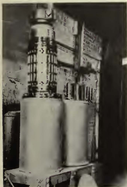
[ At left ] Removal of armature coils is facilitated by soaking in a hot cleaning solution for several hours
