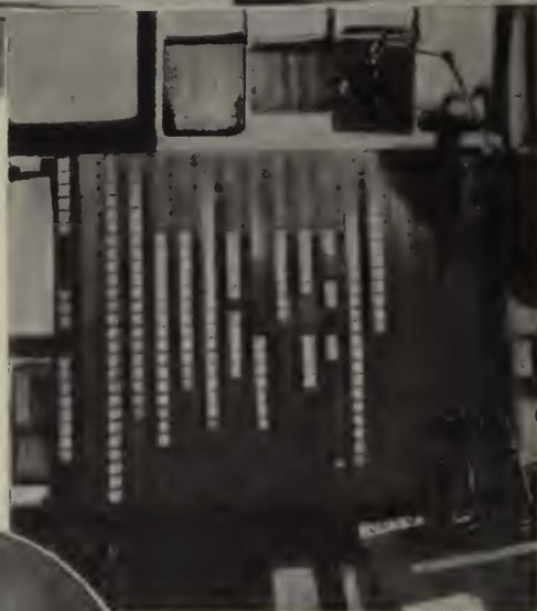
Plug board used by the dispatcher in assigning buses for the day's run
