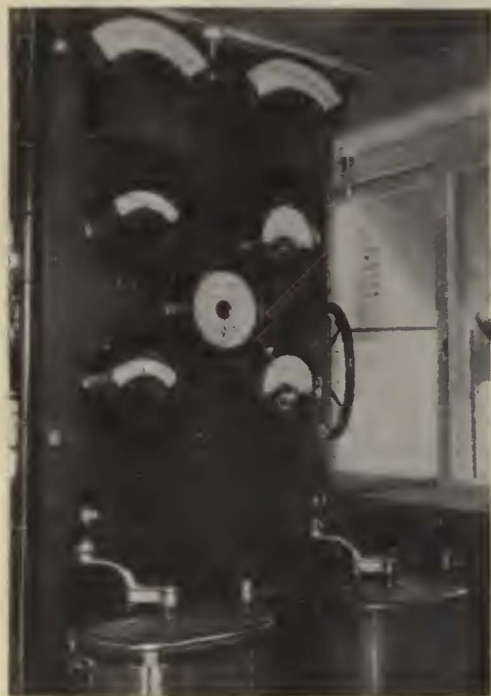
Switchboard and controllers for test performance are inclosed in booth alongside of stand
