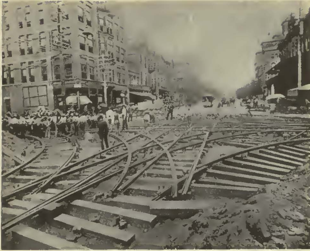
Typical track construction of the early '90's. "Bolted Up" special trackwork on chairs laid in Atlanta, Georgia, 1891
