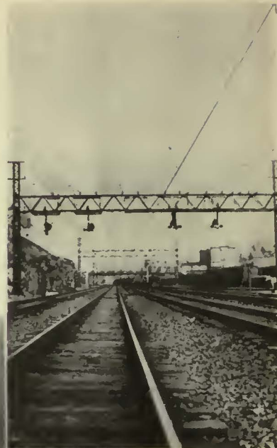
Typical installation of overhead catenary on the Pennsylvania Railroad between Philadelphia and Wilmington. The type now being installed on other sections is quite similar
