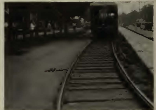
Temporary track construction with Bethlehem No. 3-A Steel Ties equipped with special base plates.
