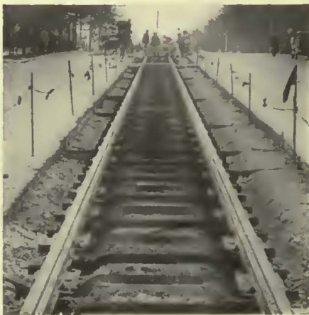
In the Washington, D. C., standard, adopted in 1929, the concrete pavement is practically the sole support of the rails
