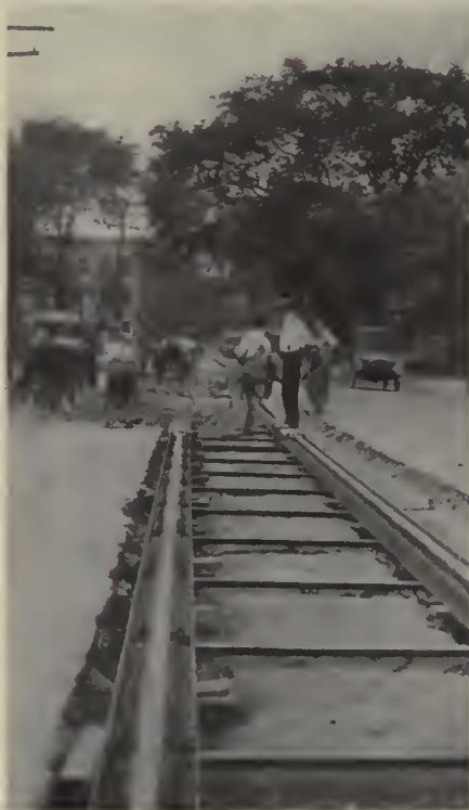
New type "quiet" track, using concrete-embedded channels in which an asphaltic concrete is tamped around the rail
