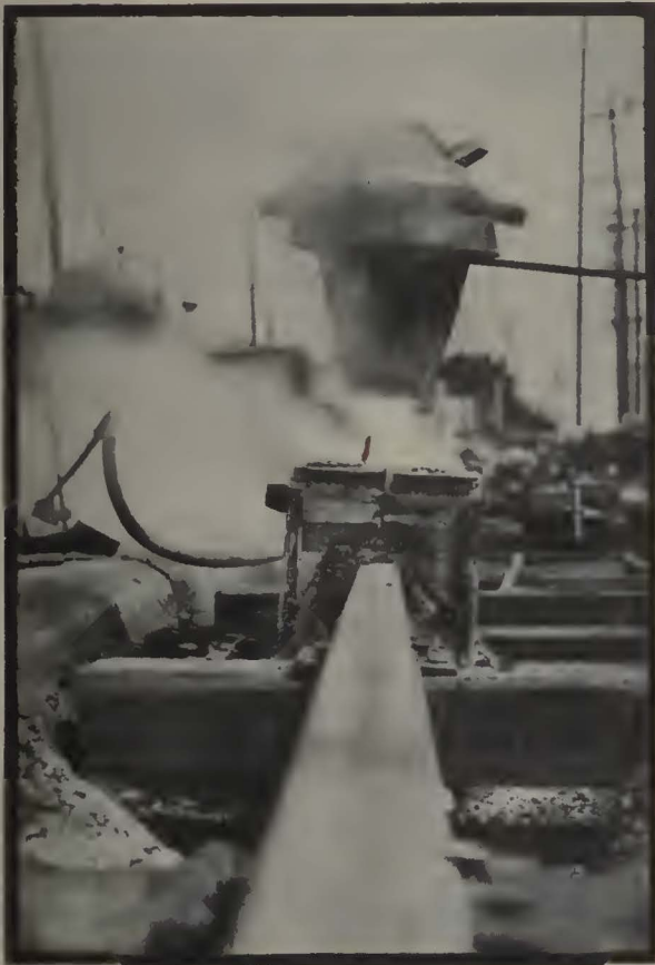
Pouring a Thermit weld, with 80 lb. A.S.C.E. rail in East Point line, Atlanta.
