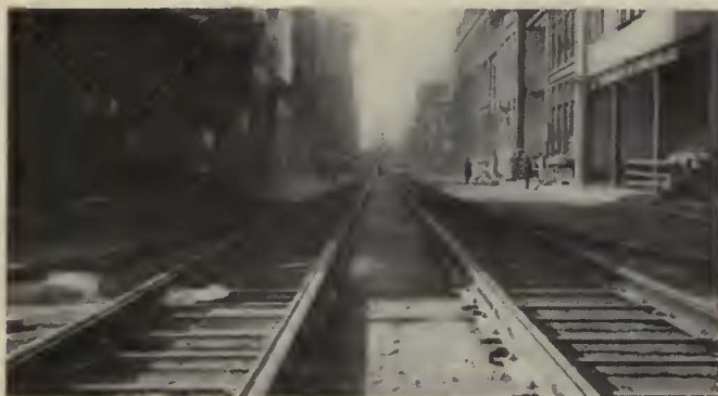
International steel twin ties were installed when this double track was rebuilt
