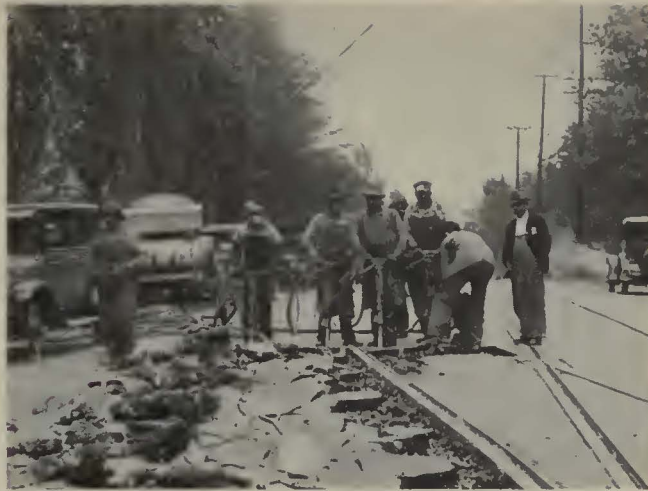
Pneumatic paving breakers and other modern machines help the roadway department to lower costs
