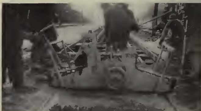
Through use of International concrete pulsator track now can be built under service
