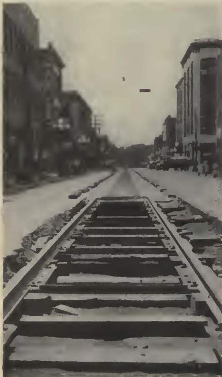
In reconstructing this track the old wood ties were left in place and steel ties placed between them
