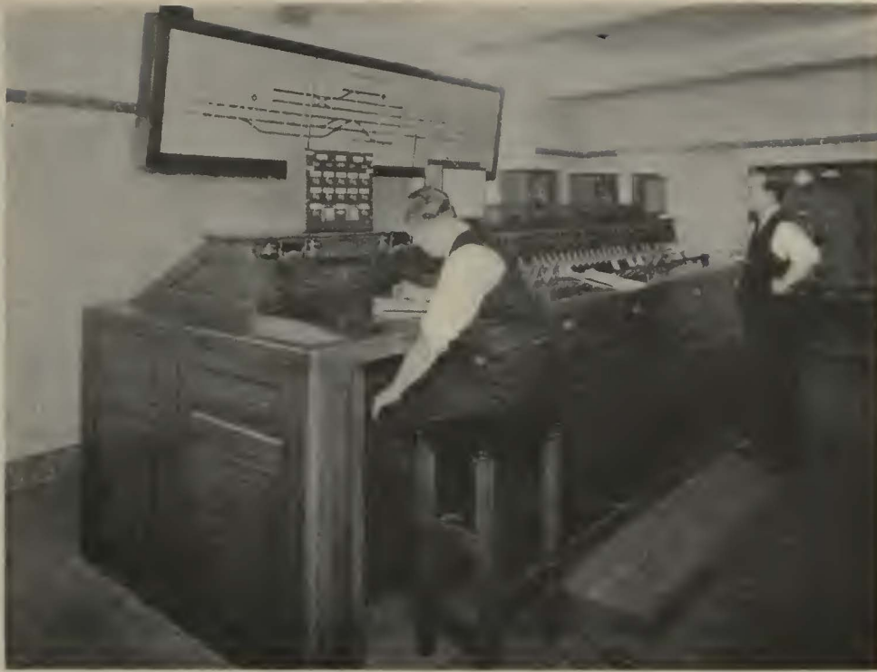
Interlocking connections at the Hammersmith Station in London are controlled from this board
