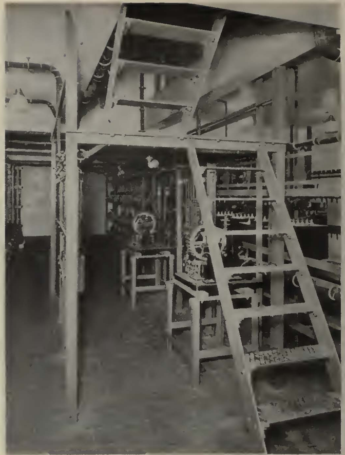
The relay room is directly beneath the signal cabin. A ladder leads to the gallery below the control board
