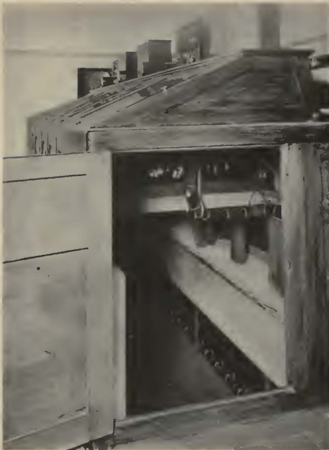
Access to a gallery beneath the board is obtained through a door in the end of the cabinet
