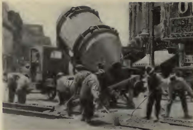
Premixed concrete was used for the paving base with asphalt for the surface
