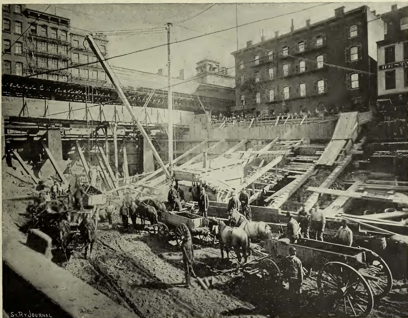
EXCAVATION AT CORNER OF BAYARD STREET AND BOWERY, NEW YORK, FOR THIRD AVENUE CABLE RAILWAY STATION.
