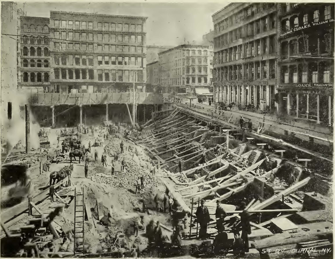
EXCAVATION AT BROADWAY AND HOUSTON STREET, NEW YORK, FOR CABLE POWER STATION.
