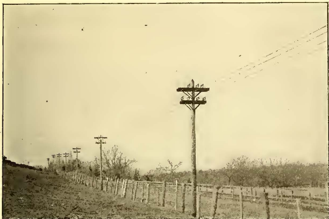
FIG. 5.—PORTION OF LINE—TAFTVILLE TRANSMISSION PLANT.
