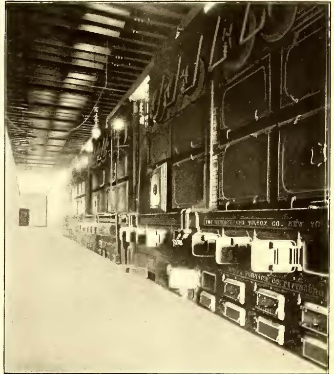
INTERIOR OF BOILER ROOM
