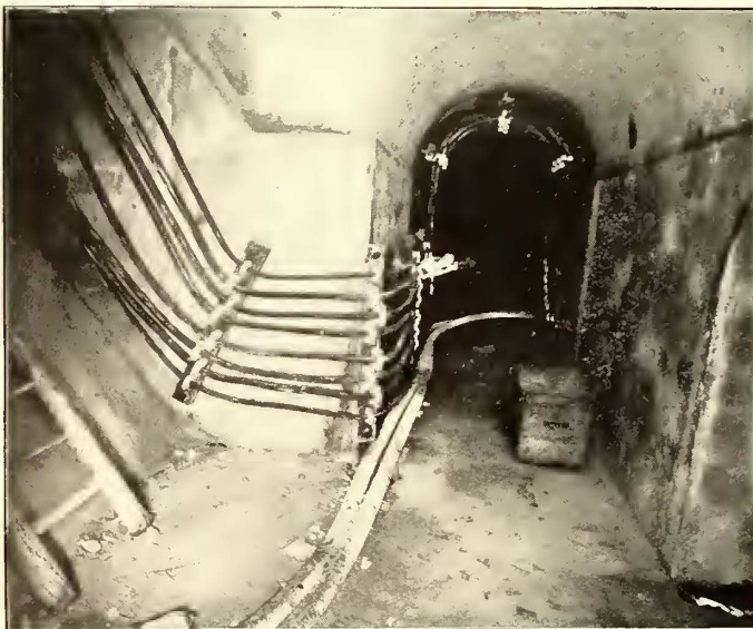
FIG. 10.—CABLE VAULTS AND GALLERIES AT PLACE DE L'ETOILE
