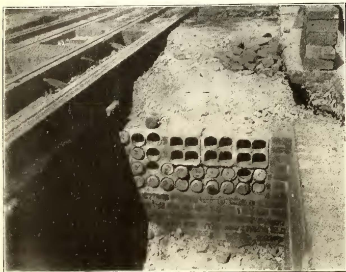
MANHOLE AND CONDUITS
