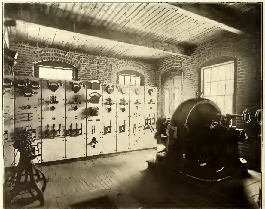
ROTARY AND SWITCHBOARD IN SUB-STATION
