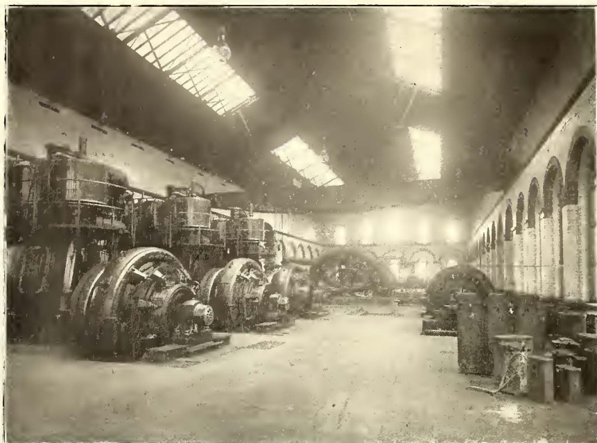
FIG. 2.—GENERAL VIEW OF INTERIOR OF POWER STATION, HALIFAX
