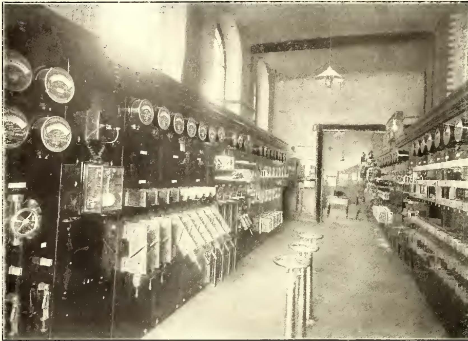
FIG. 8.—DIRECT CURRENT SWITCHBOARD AT MAIN STATION
