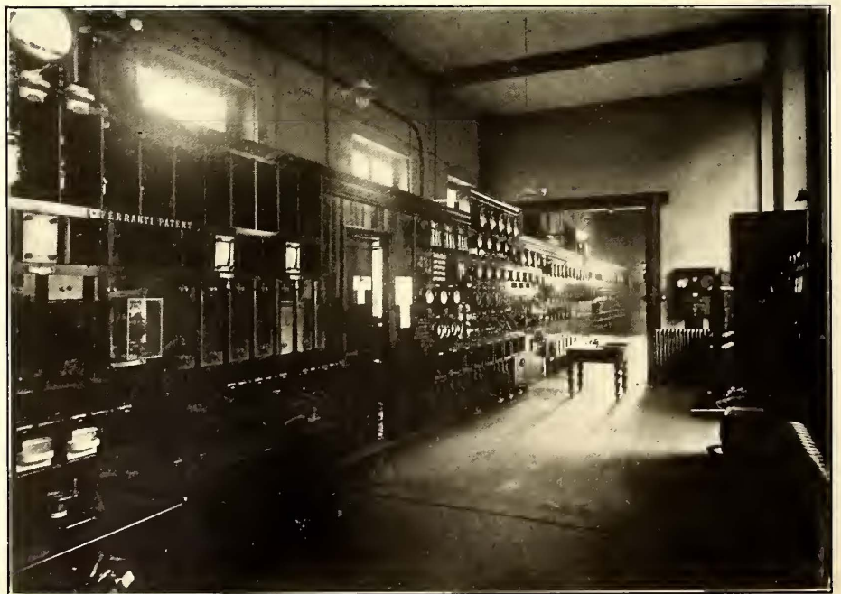
FIG. 7.—THREE-PHASE SWITCHBOARD IN POWER STATION
