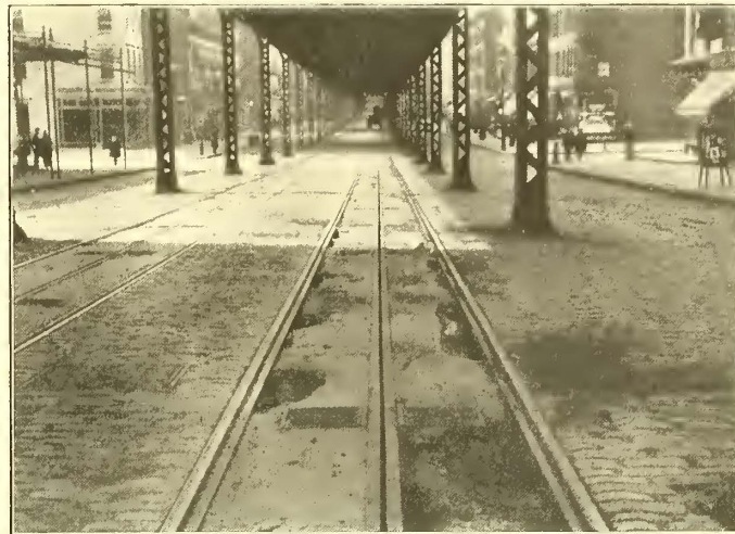
FIG. 2.—BROKEN ASPHALT PAVEMENT
