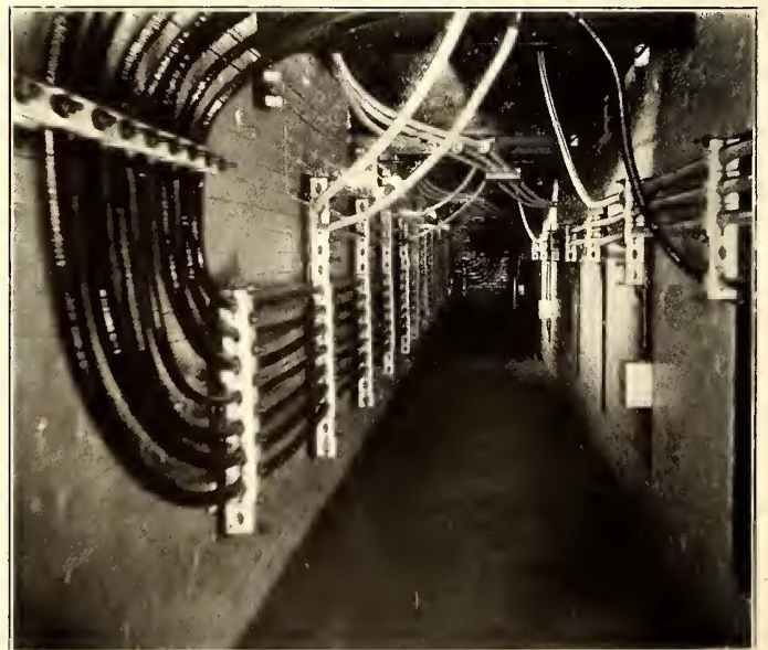
CABLEWAY IN SUB-STATION AT JOHNSTOWN
