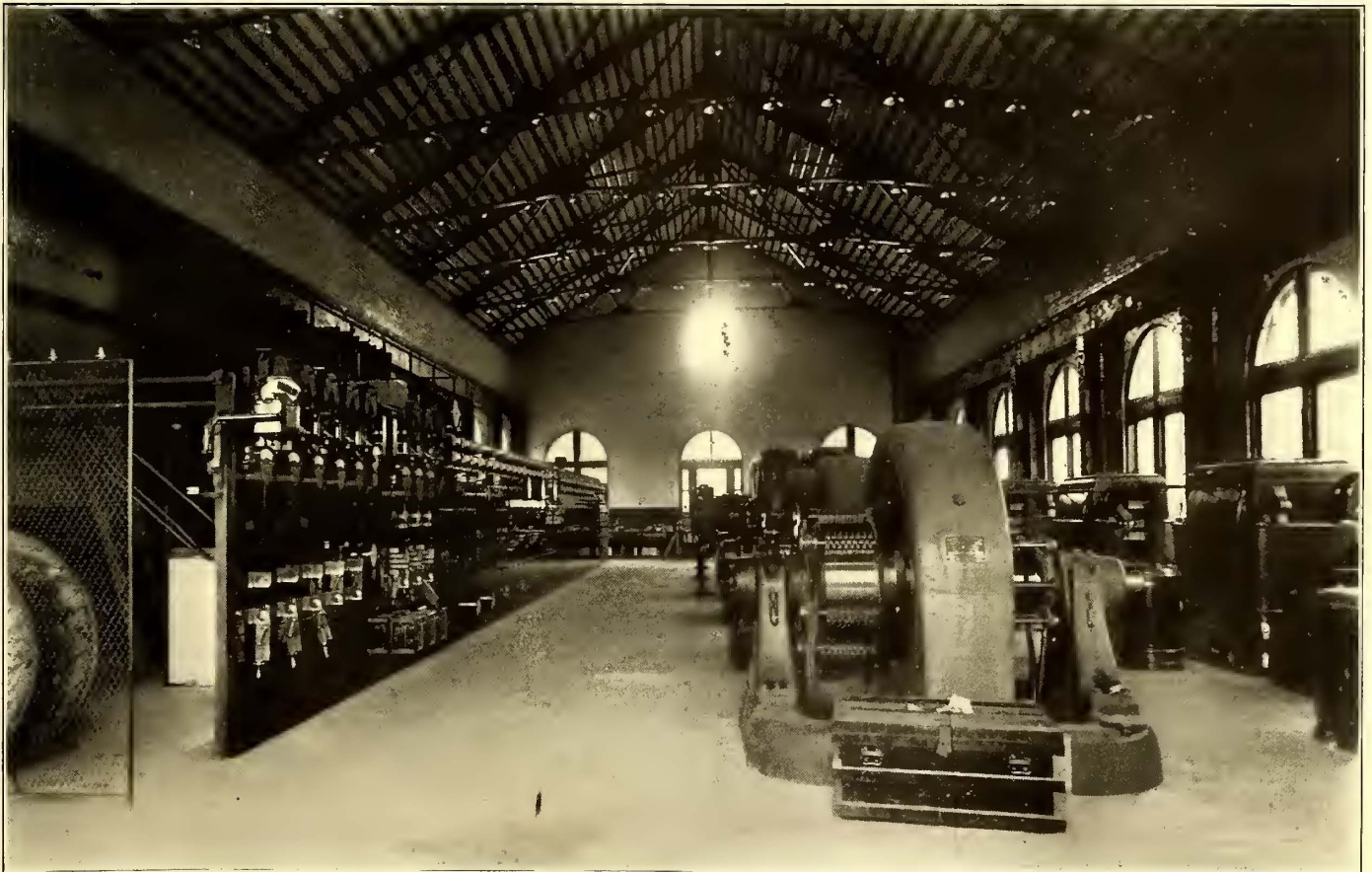
RÖTARIES, TRANSFORMERS AND SWITCHBOARD IN AMSTERDAM SUB-STATION
