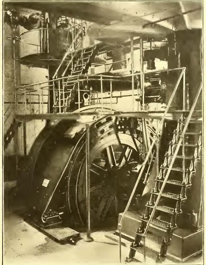
ONE OF THE 1000 KW. UNITS IN MAIN POWER STATION
