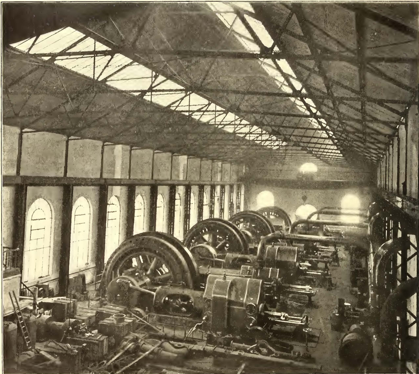
GENERAL VIEW OF INTERIOR OF POWER STATION
