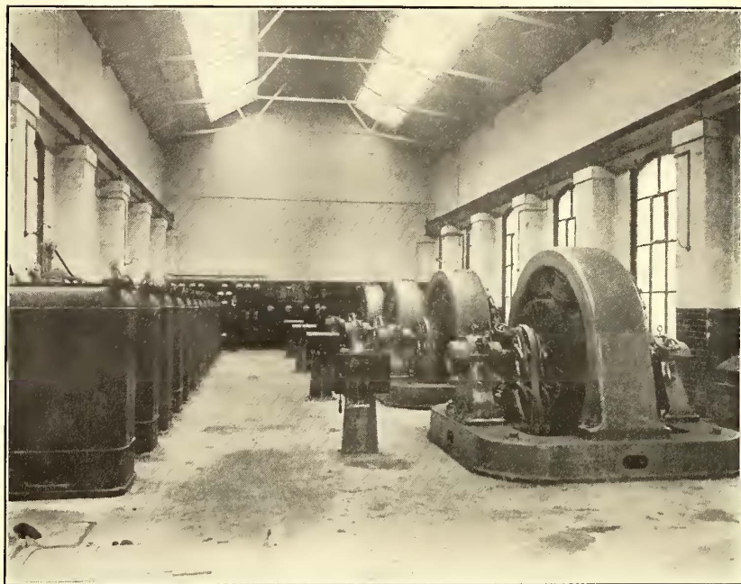
GENERAL VIEW OF INTERIOR OF SUB-STATION
