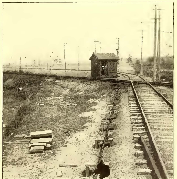
GRADE CROSSING PROTECTED BY INTERLOCKER ON CLEVELAND, PAINESVILLE & ASHTABULA RAILWAY AND NICKEL PLATE RAILROAD
