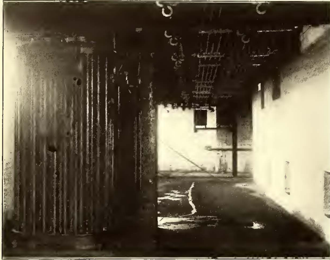
TRANSFORMERS AND WIRING IN BASEMENT OF POWER STATION
