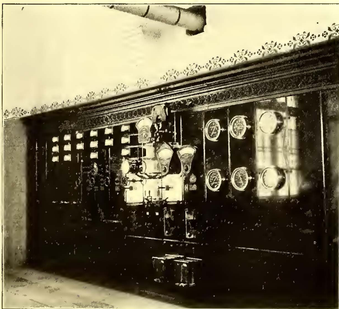
SWITCHBOARD BUILT INTO WALL
