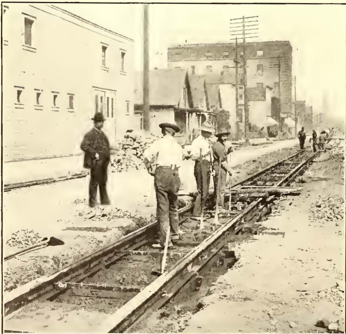
FIG. 13.—MAKING THE BED FOR THE PAVING BLOCKS AND LAYING NEW TRACK ON CONCRETE STRINGERS
