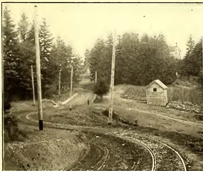
FIG. 9.—DOUBLES CURVE ON LOOP OF PORTLAND HEIGHTS LINE, ILLUSTRATING SOME OF THE SPECIAL-TRACK CONSTRUCTION NECESSARY ON THIS DIVISION
