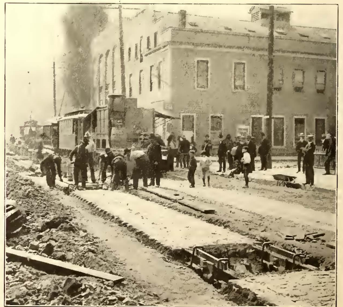
FIG. 15.—FINISHED SECTION OF TRACK AND CAST-WELDING OF JOINTS ON EAST TRACK ONLY
