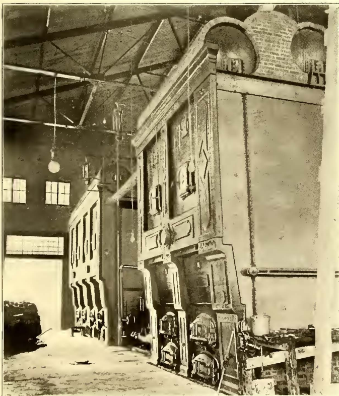
A VIEW IN THE BOILER ROOM
