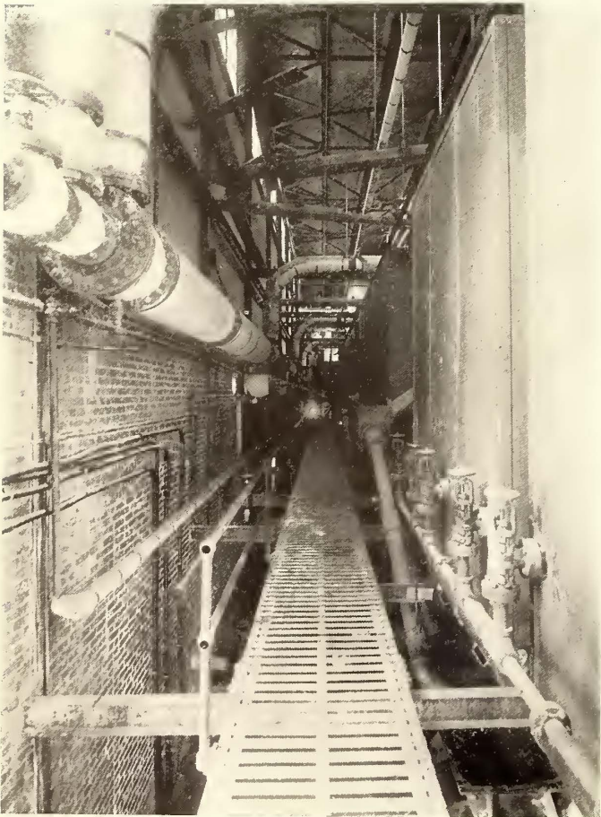
REAR VIEW OF DOUBLE-END BOILERS AT SECOND STREET AND WYOMING AVENUE STATION
