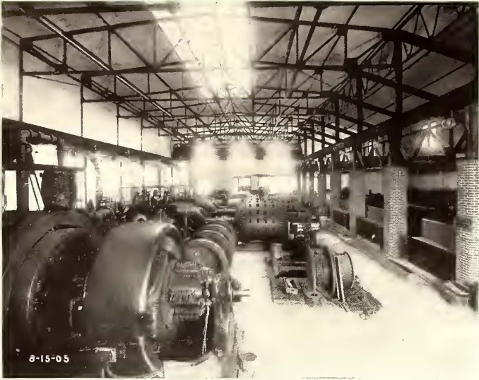
INTERIOR VIEW IN TURBINE ROOM OF GENERATING STATION AT SECOND STREET AND WYOMING AVENUE
