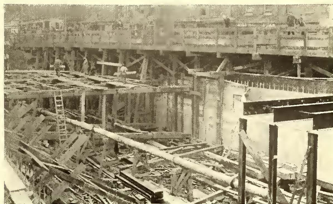
VIEW SHOWING METHOD OF SUPPORTING TEMPORARY TRACK FOR SURFACE CARS, 12-IN. CITY HALL WATER MAIN SUPPORTED AS SHOWN
