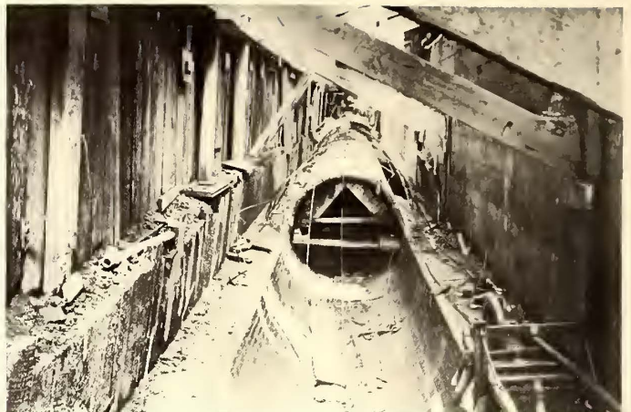
REINFORCED CONCRETE SEWER, BUILT TO REPLACE OLD SEWERS IN LINE OF SUBWAY UNDER MARKET STREET
