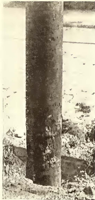
Pole with Base Badly Corroded
