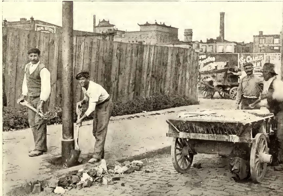
Putting in Concrete at Base of Reclaimed Pole—Portable Concrete Mixer Shown at Right RECLAIMING IRON POLES
