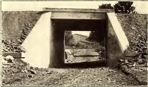
20-FT. SPAN CONCRETE STRUCTURE. DECK OF I-BEAMS IN CONCRETE. SIDE WINGS ARE ARRANGED TO AVOID FORMING A BLIND CURVE
