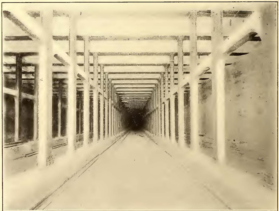
VIEW TAKEN SEPT. 26, 1905, BEFORE TRACKS WERE LAID, SHOWING REINFORCED CONCRETE STRUTS BETWEEN COLUMNS
