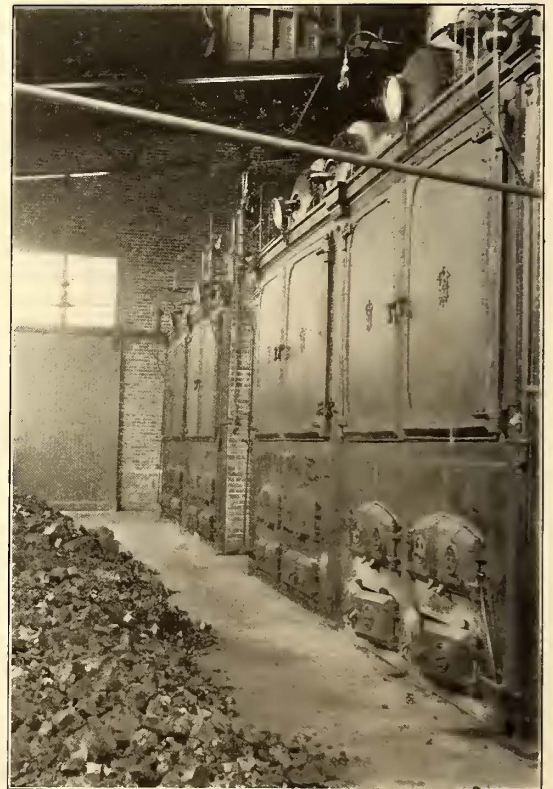
BOILER ROOM OF THE TOLEDO, PORT CLINTON & LAKESIDE RAILWAY
