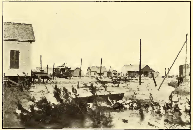
VIEW AT GALVESTON, SHOWING AREA SHORTLY AFTER IT HAD BEEN RAISED TO THE NEW GRADE
