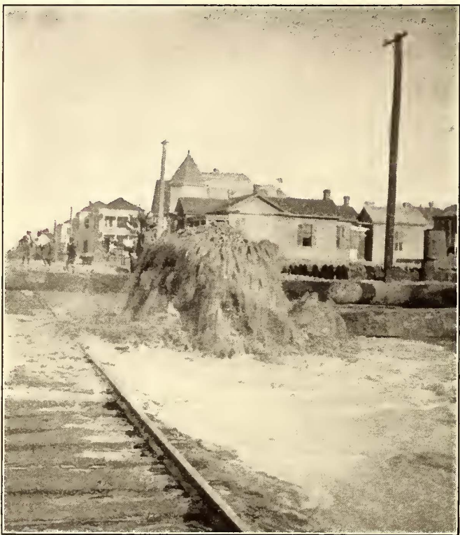
VIEW SHOWING END OF 42-IN. PIPE DISCHARGING SAND AND WATER IN THE GRADE-RAISING OPERATIONS AT GALVESTON
