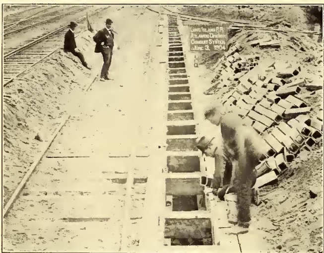
FIG. 4.—CONDUIT MANHOLES CLOSE TO TRACK, ATLANTIC DIVISION
