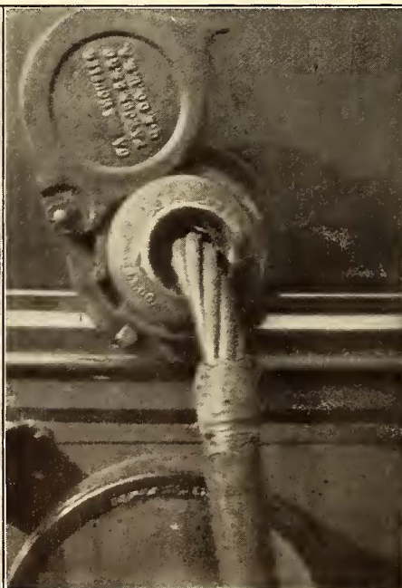
FIG. 4.—JUMPER TERMINAL WITH WIRE EXPOSED
