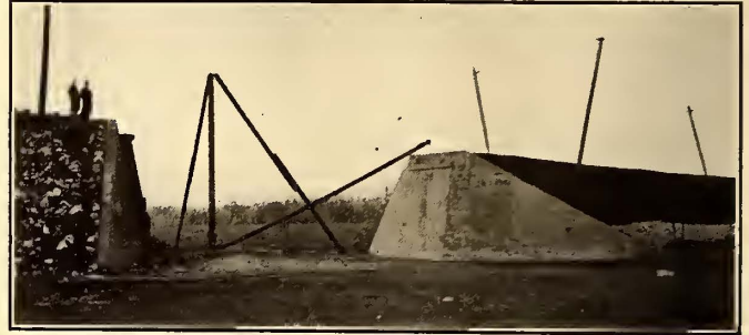
FIG. 1.—BREAK IN THE LEVEE NEAR CENTER CREEK FOR MISSOURI PACIFIC SWITCH
