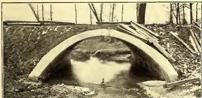
FIG. 1.—A 22-FT. HORSESHOE ARCH ON THE INDIANAPOLIS & WESTERN RAILWAY
