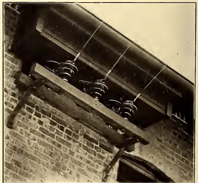
HIGH-TENSION WIRES ENTERING HERROLL SUB-STATION
