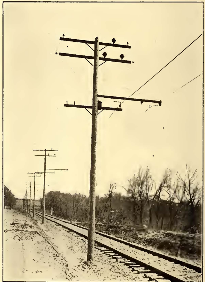
ONE OF THE SPECIAL POLES PLACED EVERY 1000 FT., UPON WHICH LIGHTNING ARRESTERS ARE GROUNDED, TROLLEY FEED-IN TAPS ARE MADE, AND THE HIGH-TENSION GROUND WIRES RUN TO EARTH
