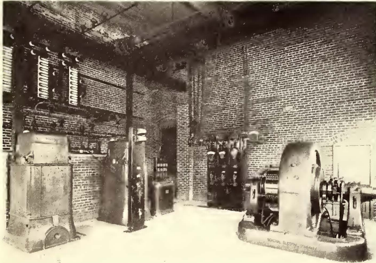
INTERIOR CHASELAND SUBSTATION, COLUMBUS, DELAWARE & MARION
