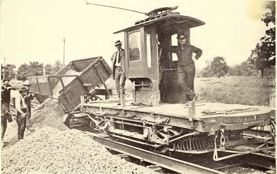
CONCRETE GIRDER CONSTRUCTION IN COLUMBUS—DELIVERING MATERIAL WITH SIDE-DUMP CARS. ONE MOTOR CAR WILL PULL TWO DUMP CARS
