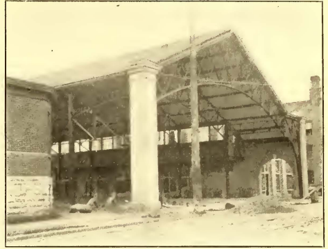
EAST CHARLES STREET FRONT OF TRAIN SHED, SHOWING CANTILEVER CONSTRUCTION OF TRUSS
