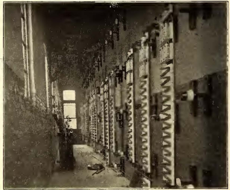
FIG. 14.—VIEW OF LIGHTNING ARRESTER ROOM, NEWFIELD SUB-STATION
