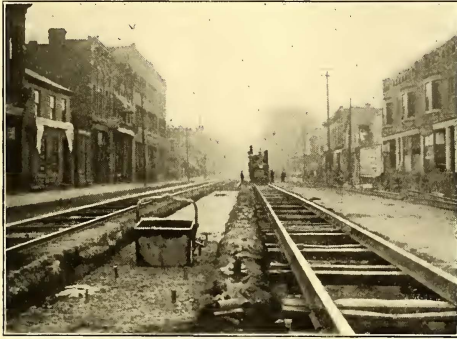
FIG. 10.—CONCRETE BED ON GRAVEL, AND TRACKS LAID UPON THIS, IN THE DISTANCE
