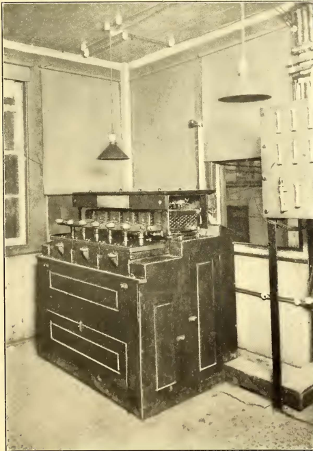
FIG. 4.—INTERIOR VIEW OF SWITCH TOWER
