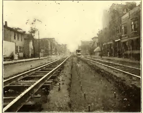
FIG. 11.—TEMPORARY TRACK ON THE RIGHT, GRAVEL BED READY FOR CONCRETE ON THE LEFT, AND TEMPORARY TRACK OVER CONCRETE ON THE LEFT
