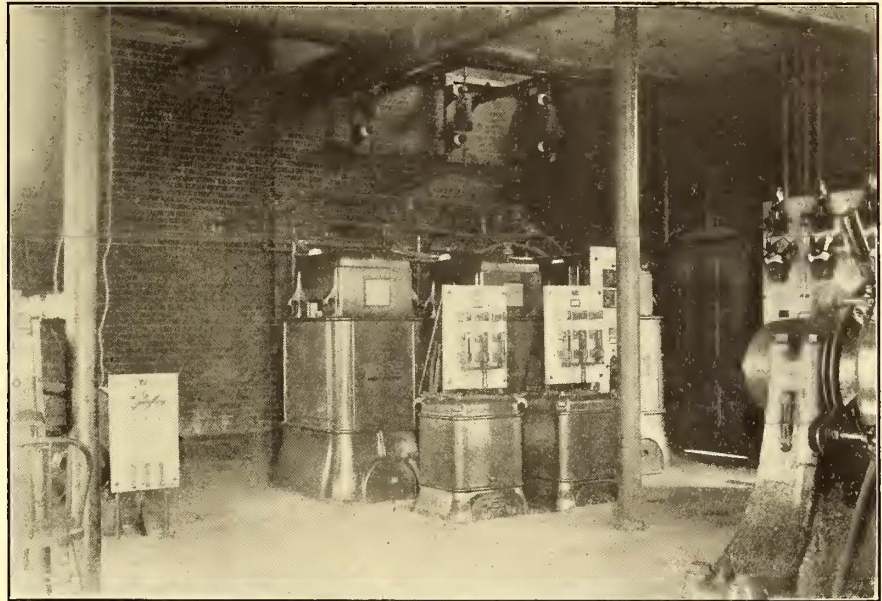
INTERIOR OF GRANITE CITY SUB-STATION, SHOWING TRANSFORMERS AND END OF THE SWITCHBOARD
