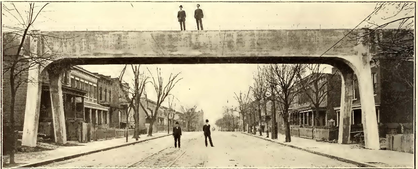
CLAY STREET SPAN COMPLETED WITHOUT TRACK. SPAN 67 FT. 5 INS. CENTER TO CENTER
