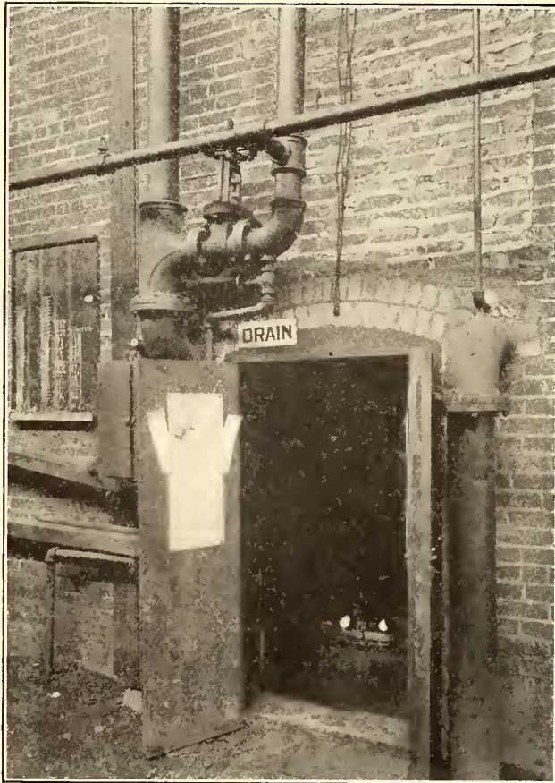
FIG. 3.—ENCLOSURE FOR VALVE WITH DOOR OPEN AND LAMPS INSIDE FOR HEATING. OUTSIDE ARE THE RISERS TO ROOF AND SIDE LINE SPRINKLER PIPES
