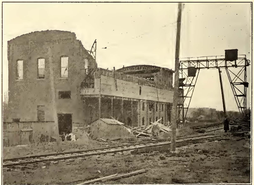
THE STATION, SHOWING THE DAMAGE TO THE ROOF AND THE ROOF TRUSSES, WHICH ARE ON THE GROUND
