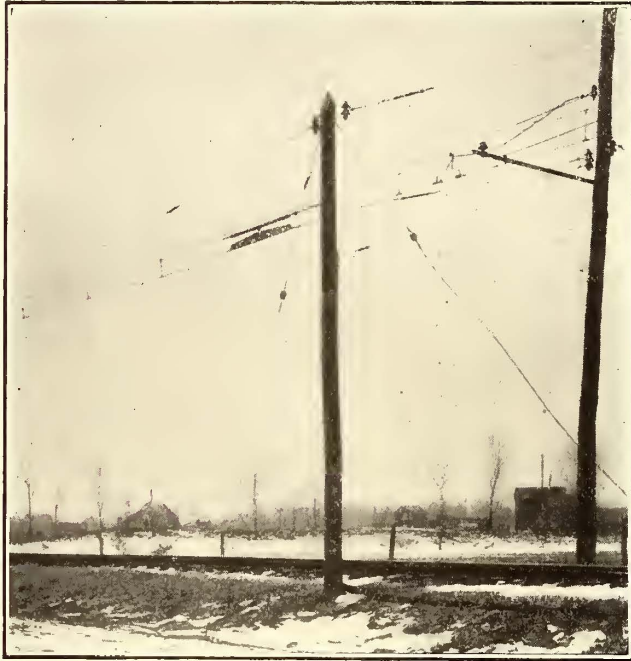
INSULATED SECTION OF TROLLEY AT DECATUR
