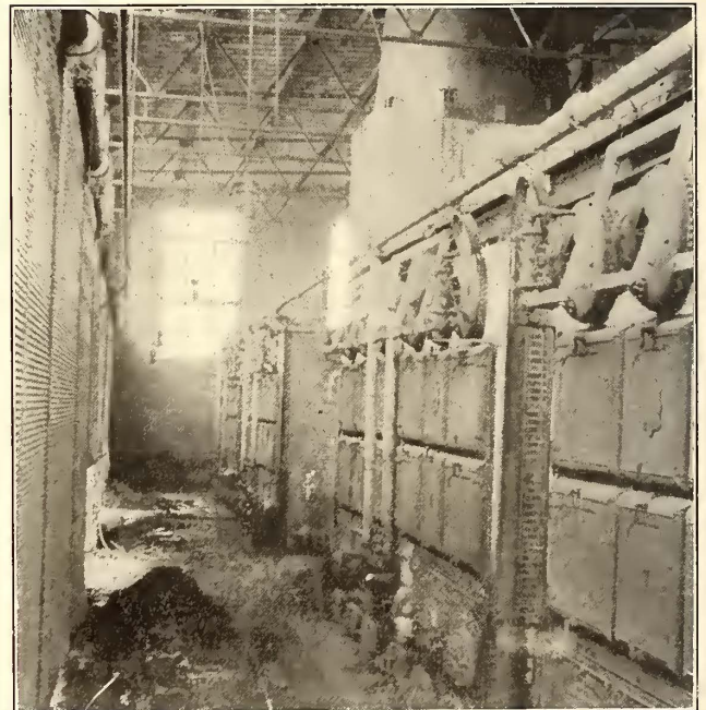
BOILER ROOM, SHOWING THE ROLLING STEEL DOORS AND METHOD OF FEEDING
