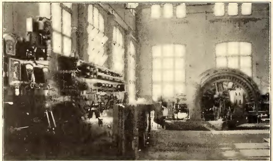
A PORTION OF THE SWITCHBOARD AND THE ROTARY CONVERTER
