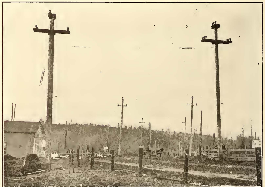
A CORNER ON THE 30,000-VOLT TRANSMISSION LINE
