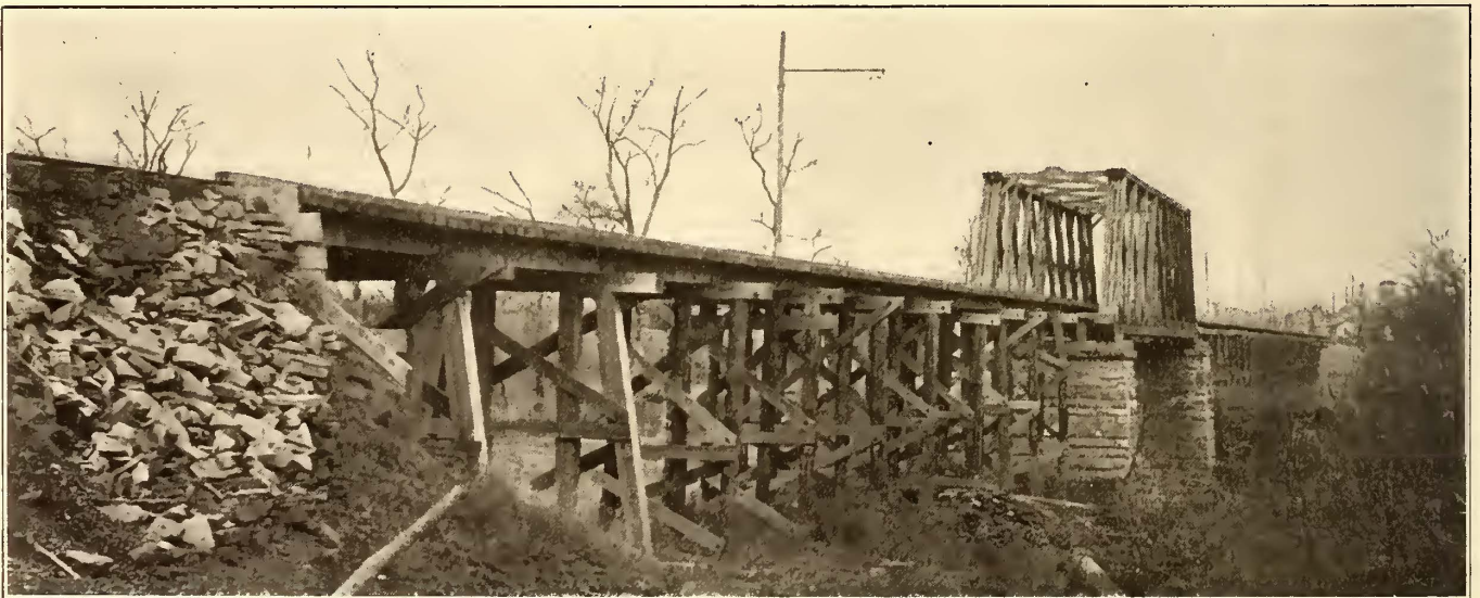
TRESTLE AND WOOD TRUSS BRIDGE AT DOW LAKE TO BE REPLACED BY A FILL
