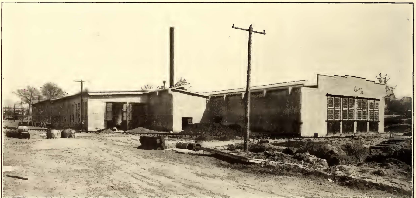
VIEW OF CAR HOUSE TAKEN FROM THE REAR TO SHOW HOW THE BUILDING WILL BE EXTENDED WHERE THE PROJECTING ROOF BEAMS ARE SHOWN
