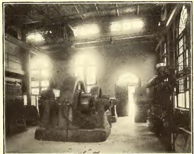
ITHAN SUB-STATION, SHOWING RELATIVE LOCATION OF SWITCHBOARD, ROTARIES AND TRANSFORMERS
