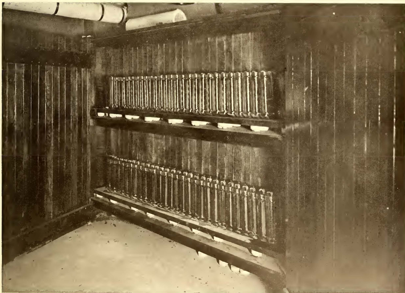
BATTERY OF CHLORIDE ACCUMULATORS FOR OPERATING OIL SWITCHES IN CLARK'S MILLS SUB-STATION, WEST SHORE RAILROAD
