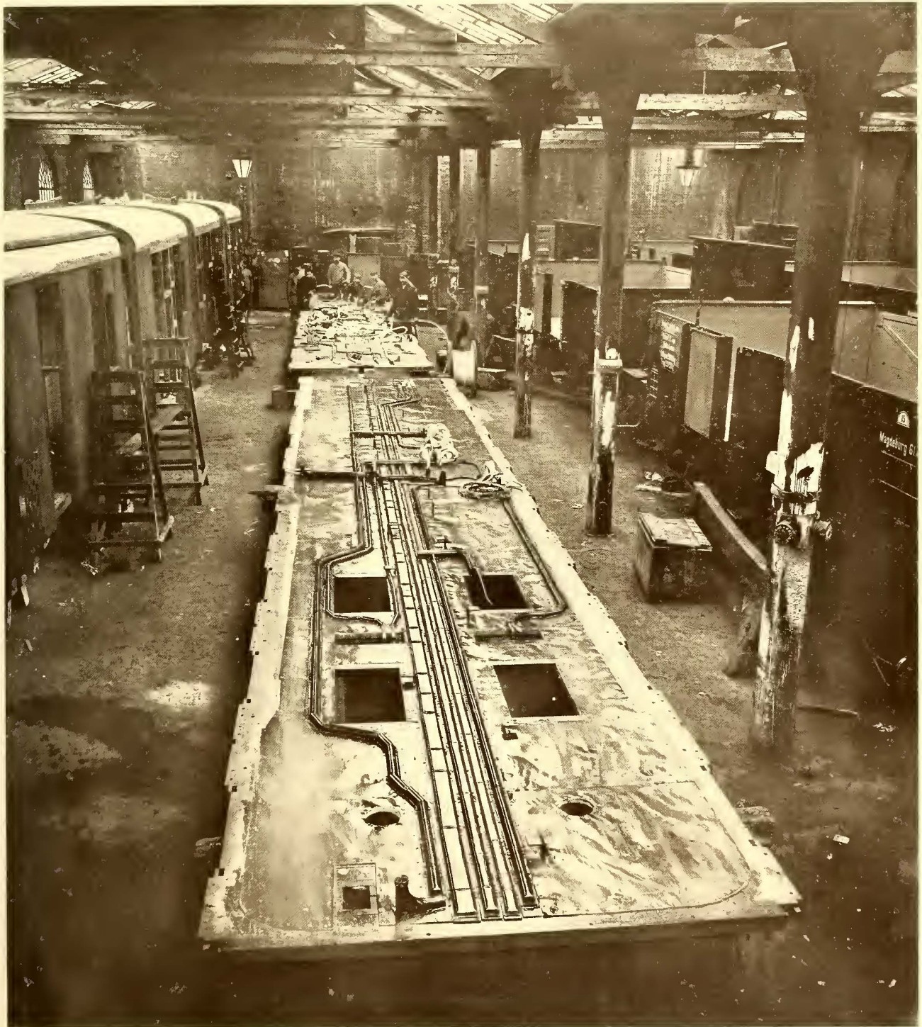
FLOOR OF HAMBURG-ALTONA SINGLE-PHASE MOTOR CAR, SHOWING HOW THE WIRING IS DONE ON THE CAR FLOORING, WHICH IS TURNED UPSIDE DOWN FOR THAT PURPOSE, BEFORE THE BODY IS BUILT INTO IT
