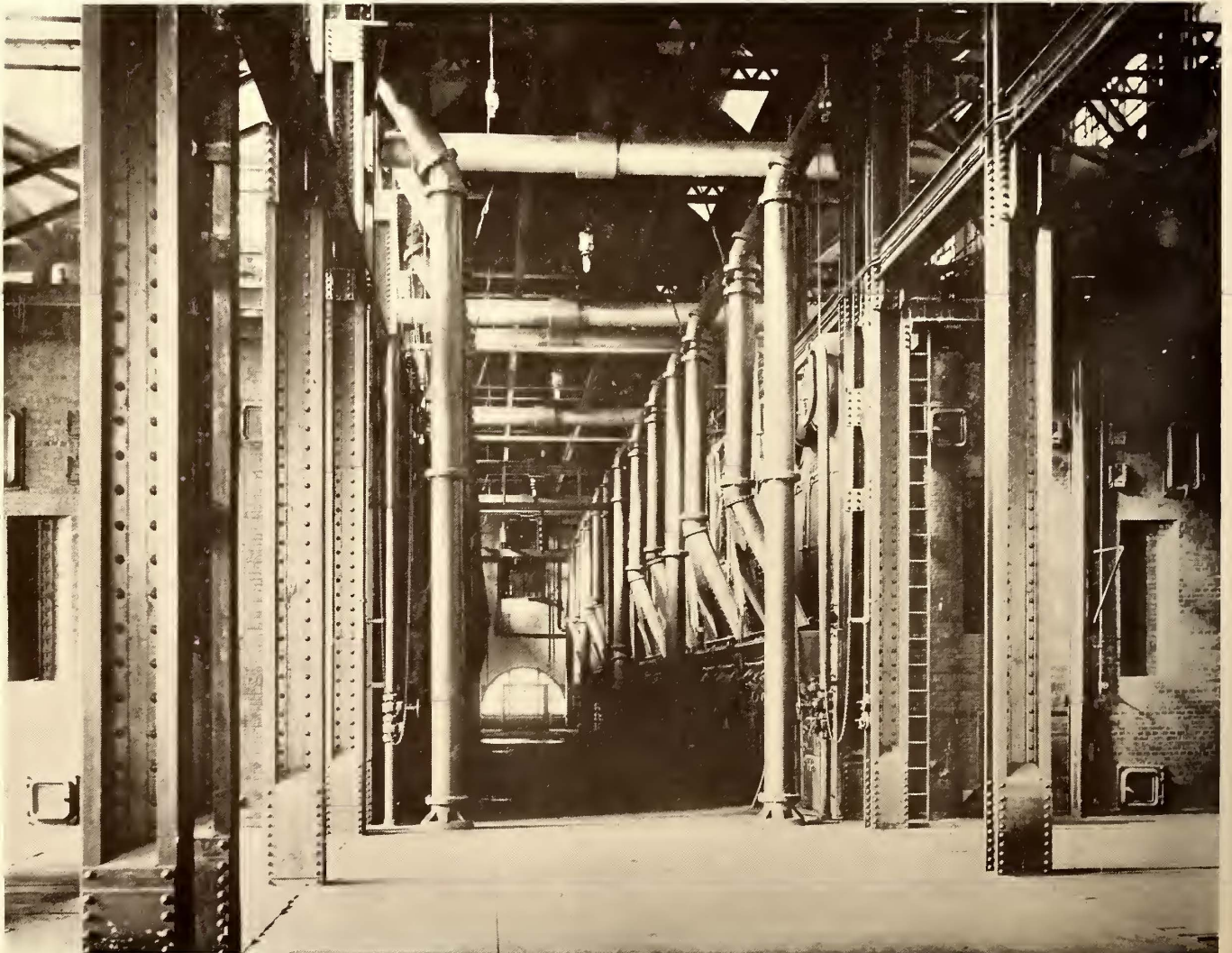
VIEW OF BOILER ROOM, LONG ISLAND CITY POWER STATION, PENNSYLVANIA TUNNEL & TERMINAL CO.
