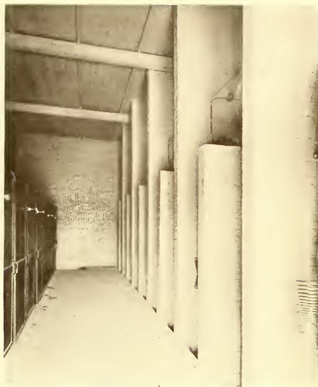
SECOND FLOOR OF HIGH TENSION COMPARTMENT, CLARK'S MILLS SUB-STATION, WEST SHORE RAILROAD
