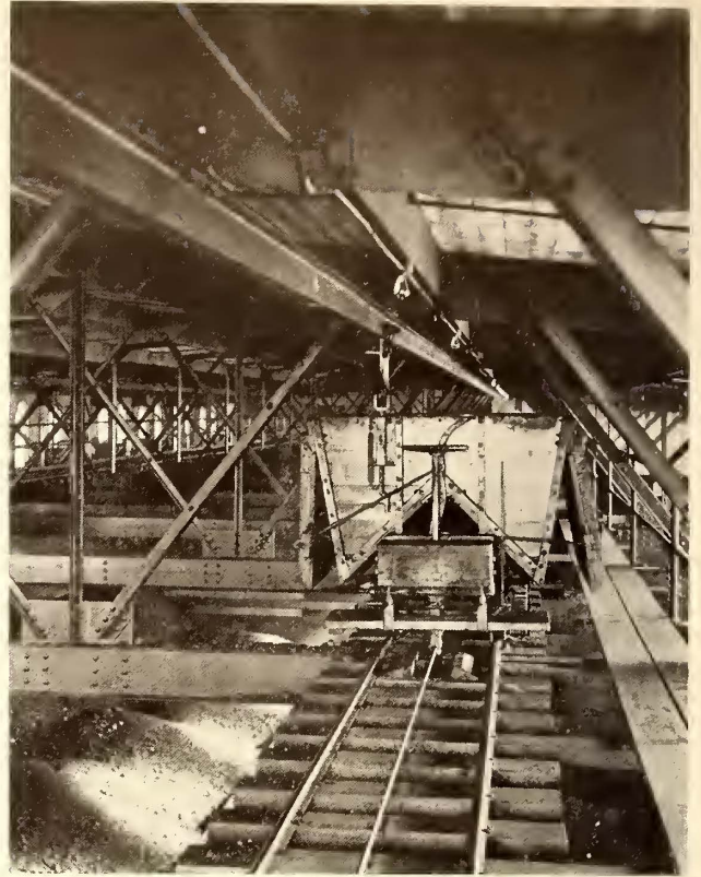
CABLE FUEL-CONVEYOR ABOVE COAL BUNKER
