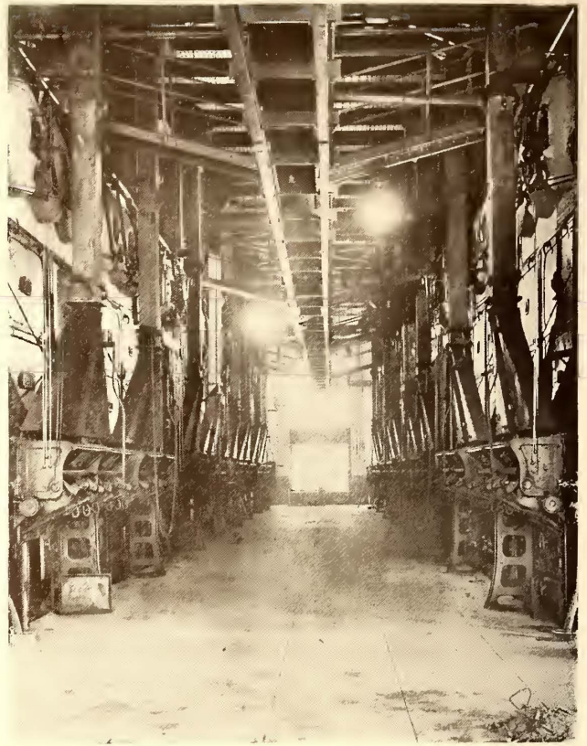
BOILER ROOM, PORT MORRIS POWER STATION
