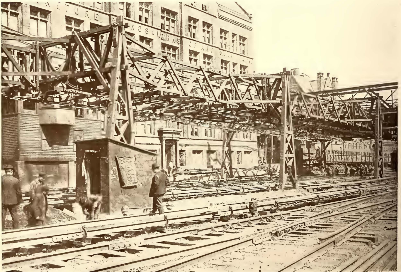
TEMPORARY OVERHEAD CONSTRUCTION IN GRAND CENTRAL YARDS BETWEEN 49TH AND 50TH STS.
