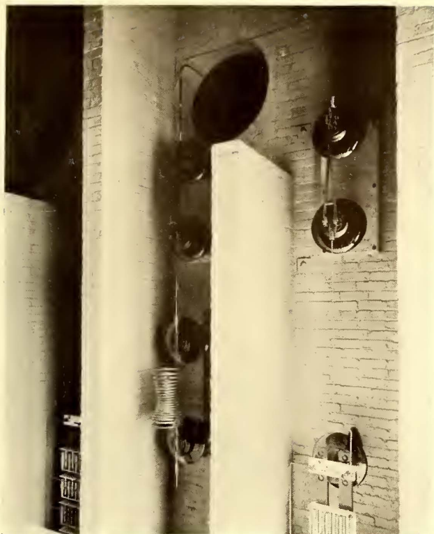
VIEW TAKEN IN HIGH-TENSION COMPARTMENT, SHOWING CHOKE COILS AND TOP OF LIGHTNING ARRESTERS, WEST SHORE RAILROAD
