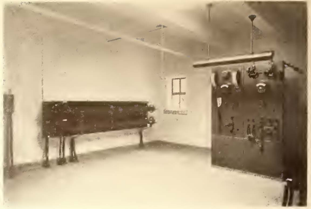
BOOSTER ROOM SHOWING BATTERY END CELL SWITCH
