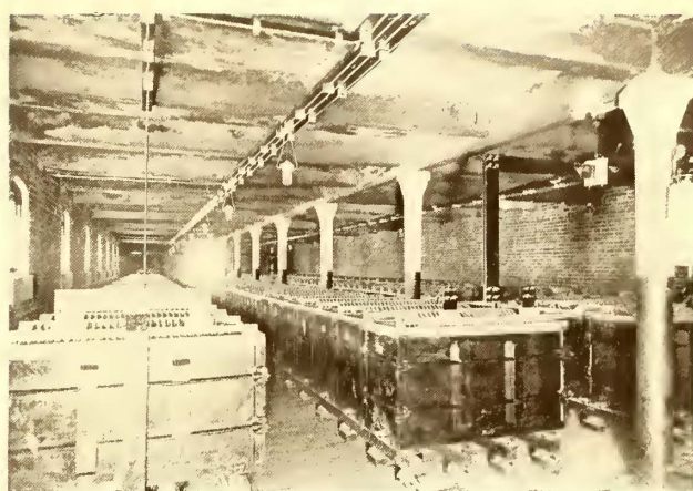
BATTERY ROOM, KINGSBRIDGE SUBSTATION
