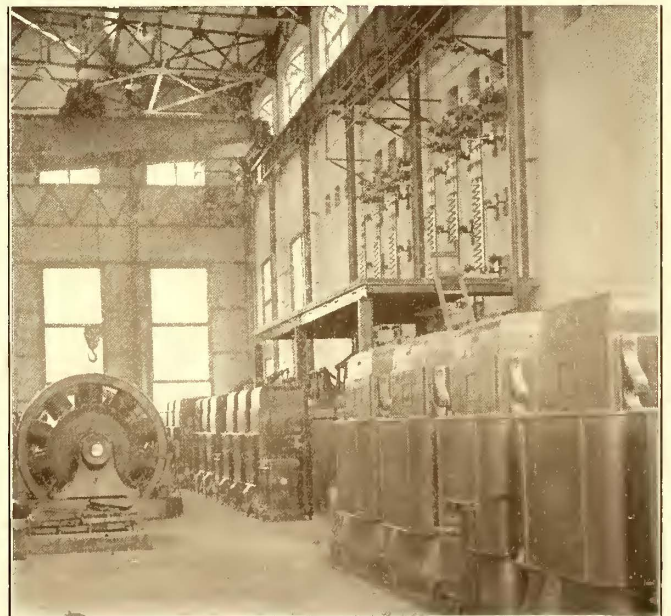
TRANSFORMERS AND LIGHTING ARRESTERS, WESTVILLE
