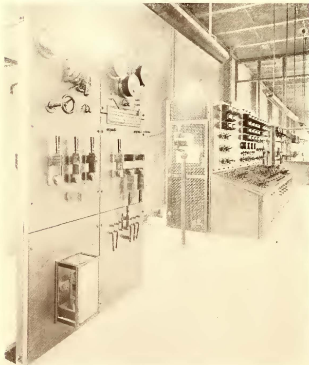
REMOTE CONTROL SWITCHBOARD
