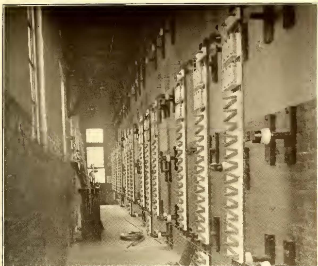
LIGHTNING ARRESTER ROOM, NEWFIELD SUBSTATION
