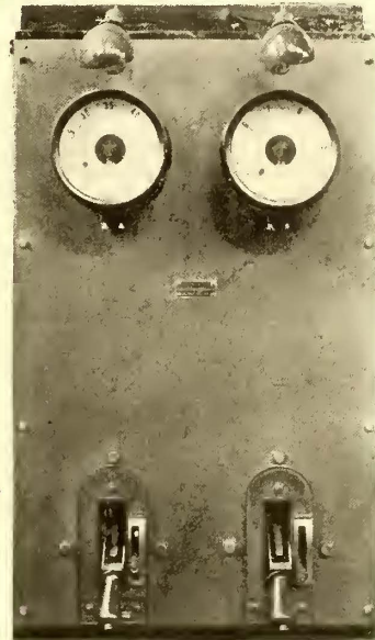
FIG. 2.—SWITCHBOARD CONTROL- LING FEEDER CIRCUIT
