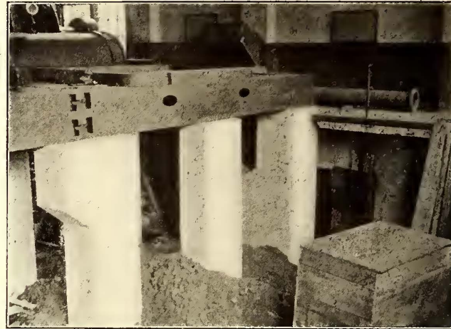
STEAM END PIERS IN WEST PENN RAILWAY COMPANY'S POWER HOUSE
