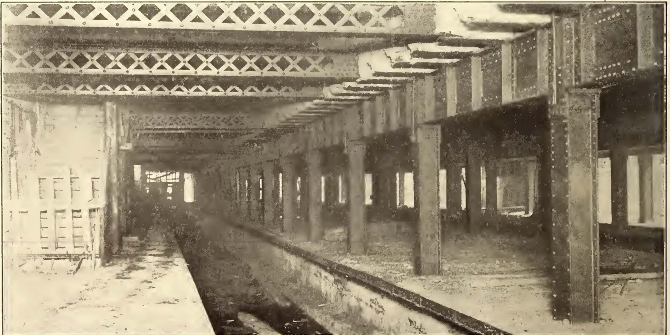
LOADING AND UNLOADING PLATFORMS FOR ELEVATED TRAINS, SHOWING WORK BEFORE TRACKS WERE LAID
