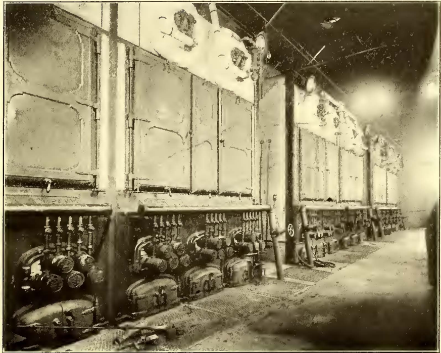
VIEW OF BOILER ROOM, SHOWING THE GAS BURNERS
