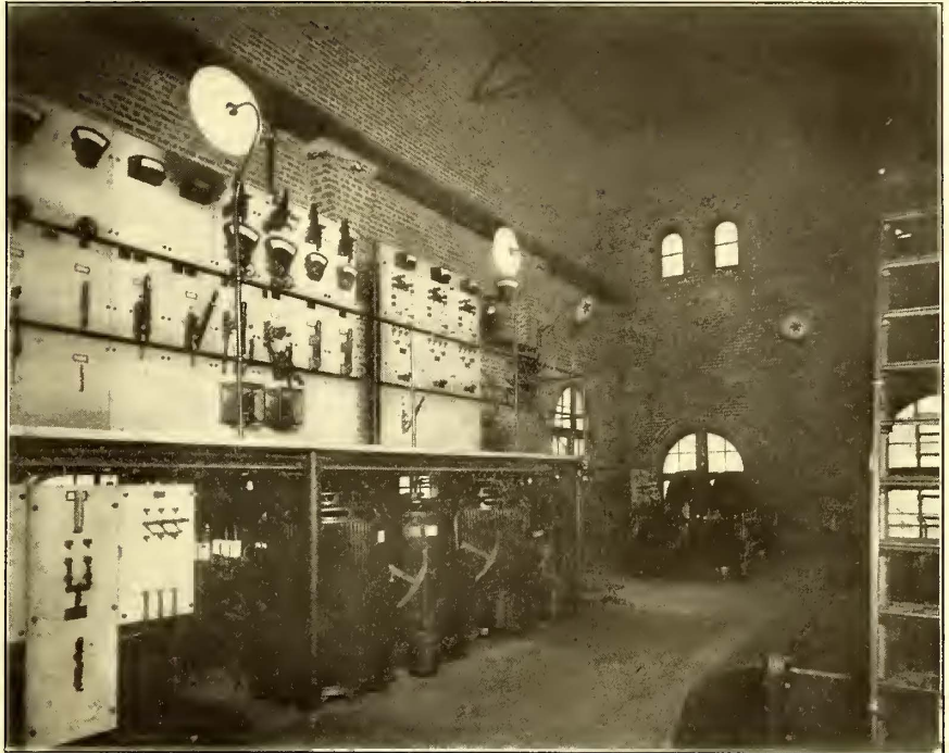
SWITCHBOARD AND TRANSFORMER VIEW
