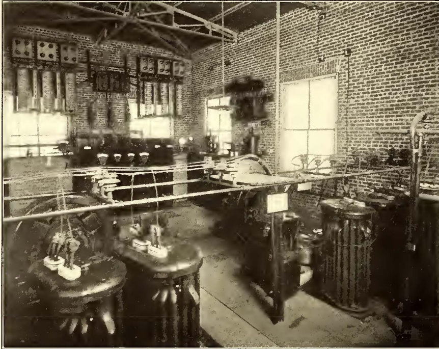
EQUIPMENT IN THE CHIEFTAIN SUBSTATION
