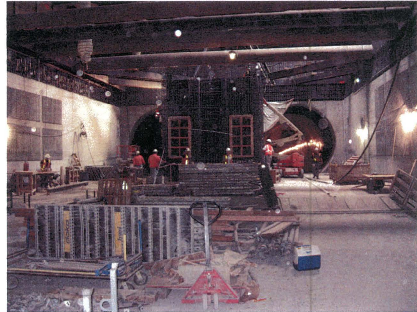
1 st /Soto Station – Work on the track level equipment rooms has begun.
