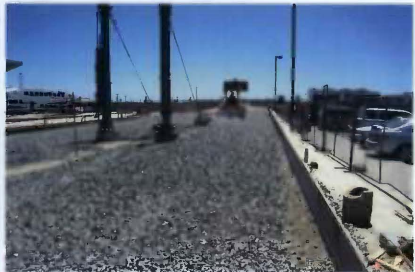
View of track ballast on the guideway looking south from Union Station towards the 101 Freeway Light Rail Transit bridge.
