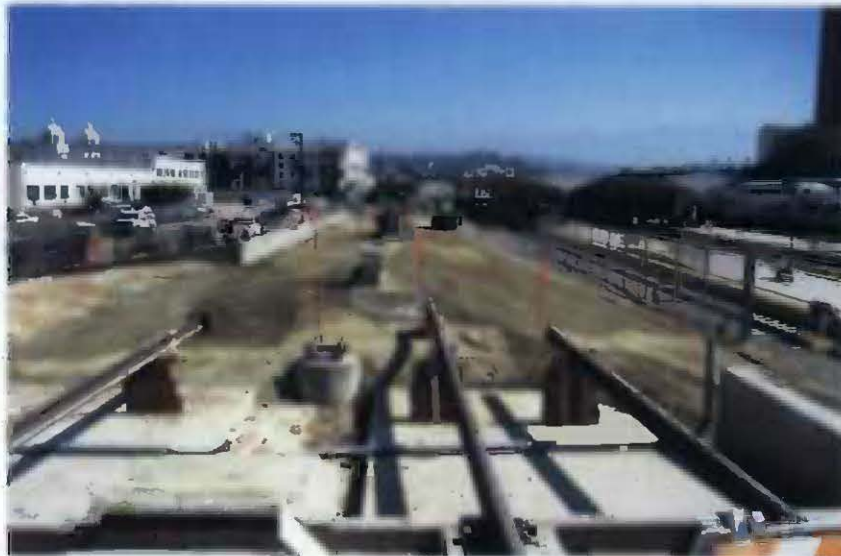
View of guideway looking north from the 101 Freeway Light Rail Transit bridge at the baggage handling road towards Union Station.
