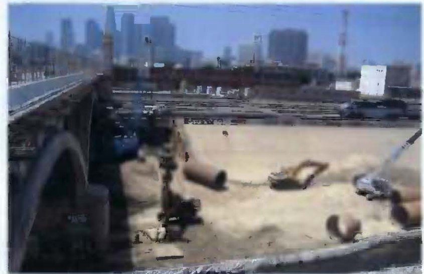
View of the City of Los Angeles Bridge Widening Project, where the bridge will be widened by 26 feet to the north.
