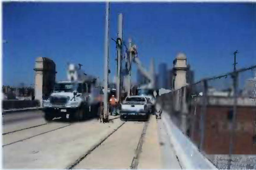
Direct current electrical cable is being fed to the LRT guideway from the traction power substation below.
