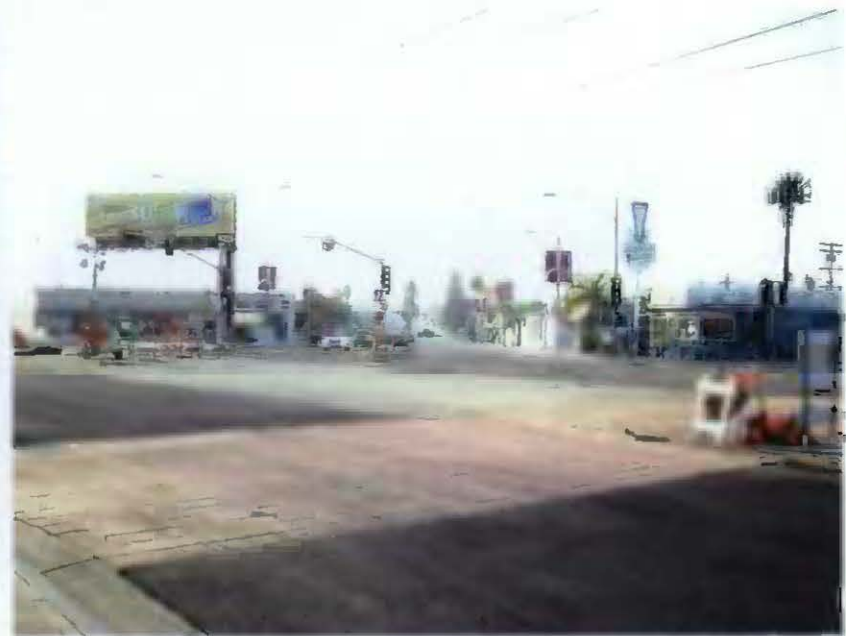
The work continues with an asphalt “overlay” for the final pavement surface.
