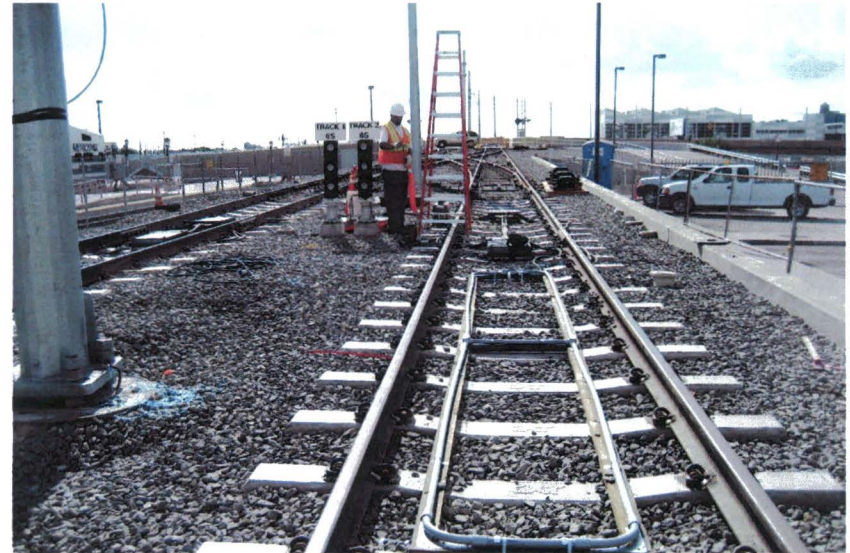
The tie-in to the Pasadena Gold Line tracks was completed in September 2008.
