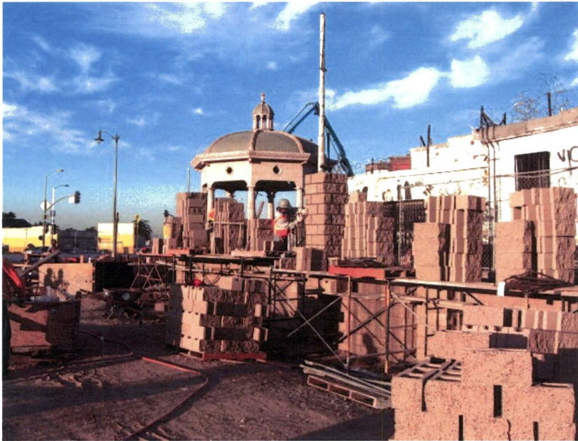
Decorative concrete masonry walls are being constructed on the plaza along the adjacent property.
