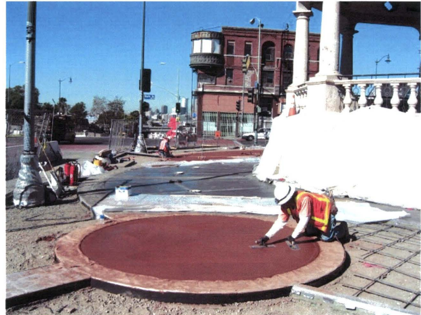
A portion of the Station Entrance Plaza near the Mariachi Kiosk being constructed prior to the November Annual Mariachi Festival.
