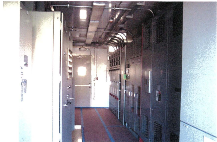
Traction Power Sub-Station 6 Interior
