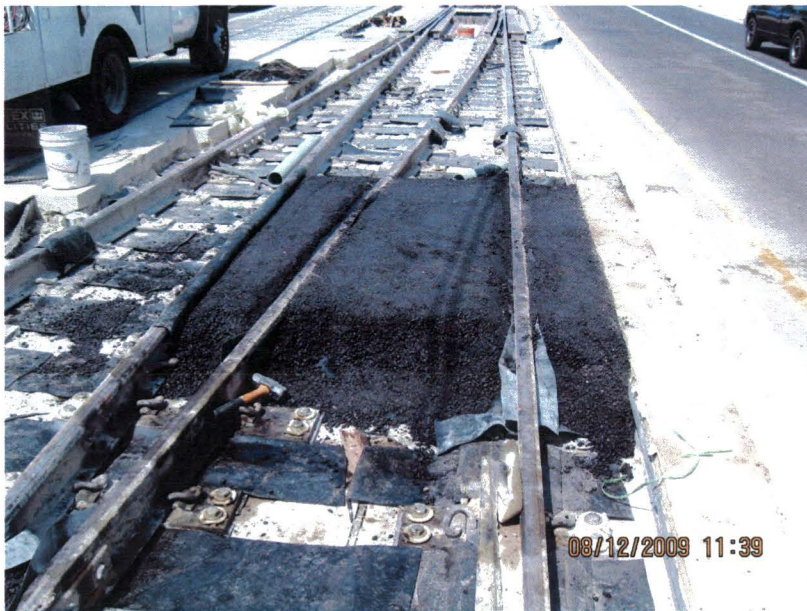
Asphalt paving and additional electrical isolation materials are being added to the crossovers to improve the train control signals.
