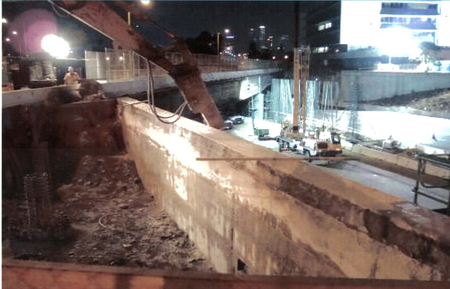
Demolition of Barrier Wall along I-110 Freeway with Bent No. 2 Rebar Installation in Background
