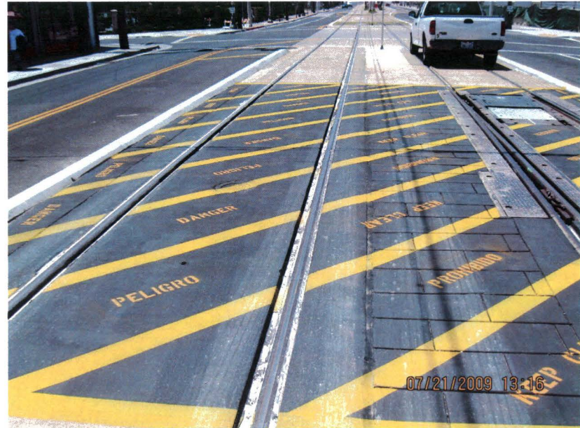
Asphalt paving color will be painted to match the colored concrete including the black areas to keep pedestrians from J-Walking.
