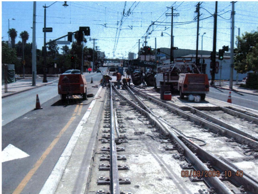
Demolition and removal of the colored concrete topping slab at 1 st /Clarence track crossover.
