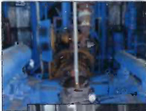
Original CNG Engine
